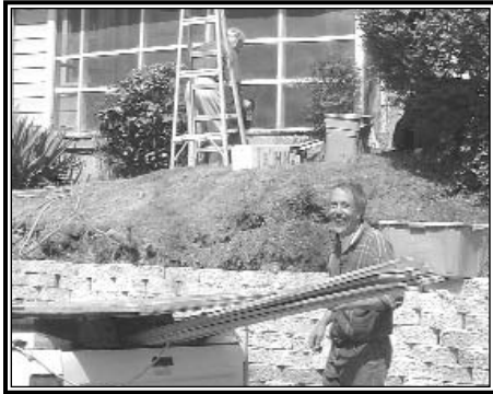
Board Member George Wright brings materials by to help rehabilitate this home at 876 Wadell Street
